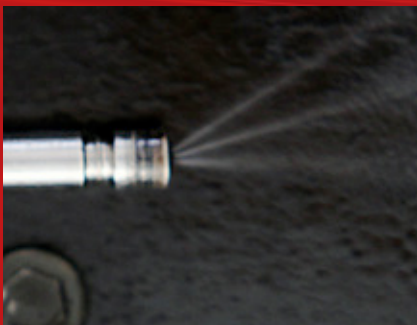
PARTIALLY BLOCKED FUEL INJECTOR
